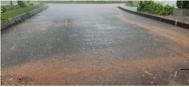
→ Bituminous Pavements generating runoff due to impervious nature
