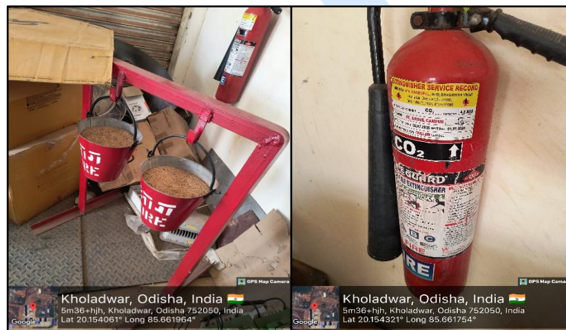
Figure 1: At Fire bucket and Fire Extinguisher at LCS
