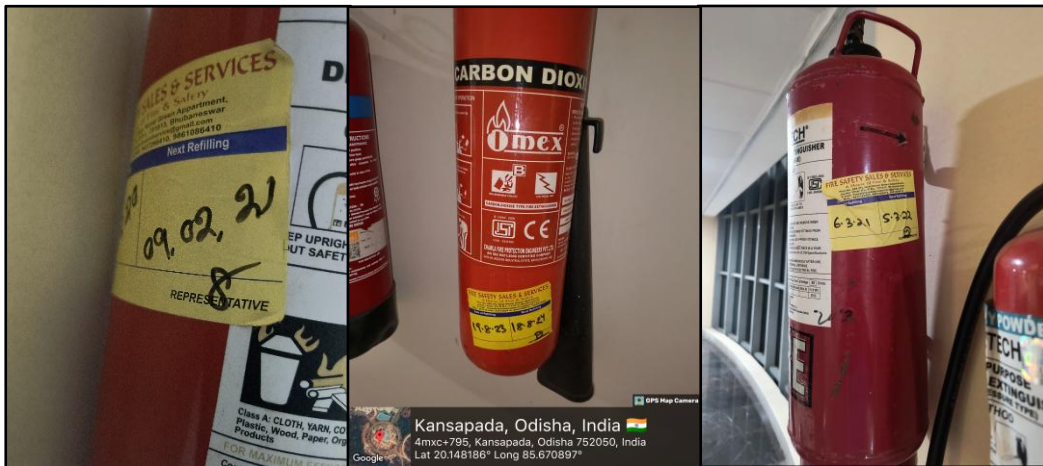
Figure 2: Expired/Due Refill Fire Extinguisher
